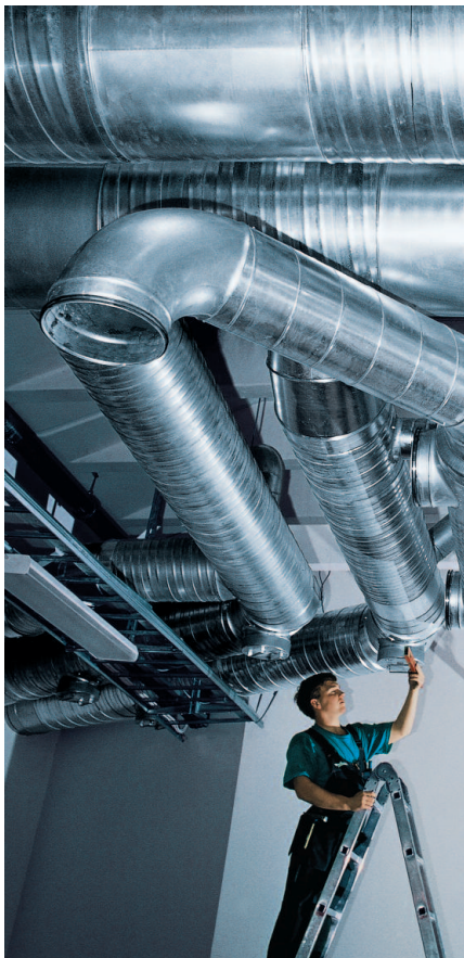
Fig. 3: Ducts made of hot-dip galvanized sheet for ventilation/air conditioning
